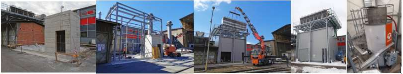
Figure 1: Electrode boiler deployment
